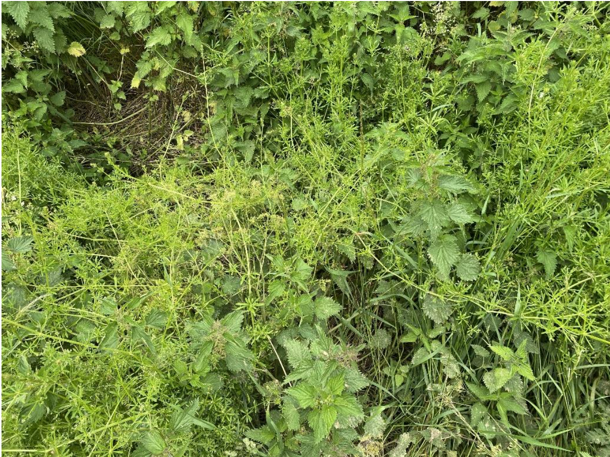
Plate 5 View of Crossing 4 ditch, choked with dense vegetation
